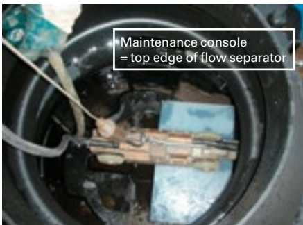
Inspection of flushing results with pan and tilt camera, camera on the maintenance console in the start shaft of a SediPipe L system
